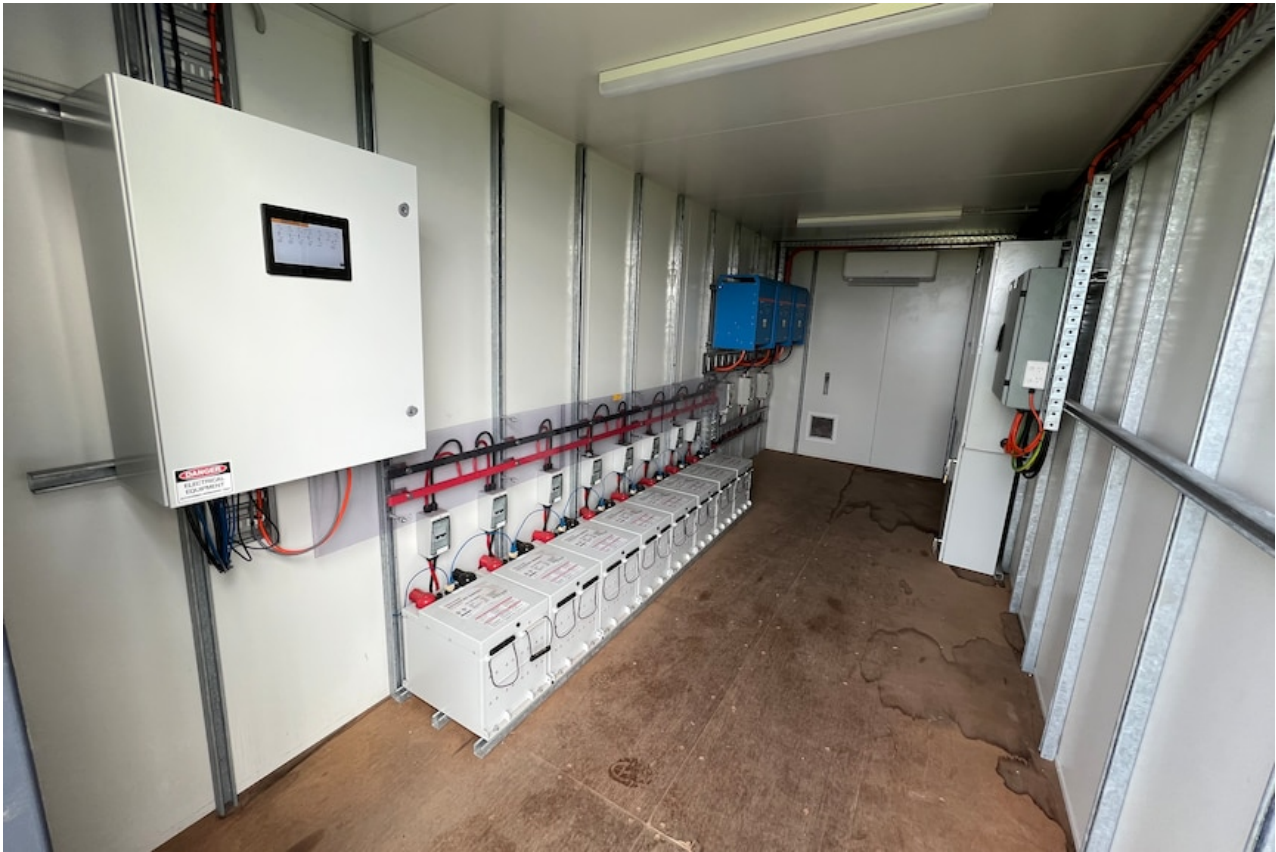
A shipping container houses inverters, batteries and a "brain" or control centre. (ABC Rural: Peter Somerville)
